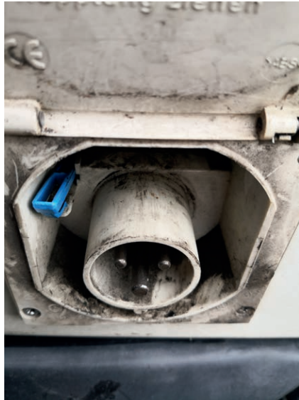
7-5. Hook-up point condition.
