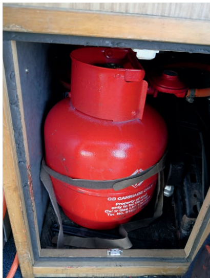
9-1. A typical gas locker compartment.
