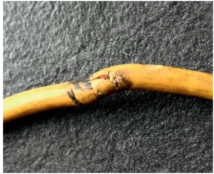
7-4. This hook-up cable has damage to the outer insulation.
