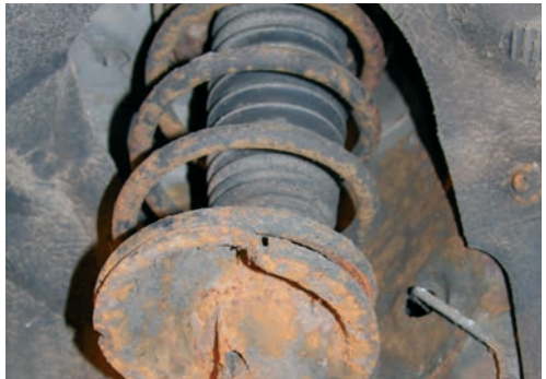
ST170 front springs have a tendency to snap, but this may not be noticed on an initial inspection.
