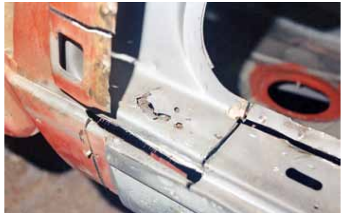
8-27. ... unlike post feet which show rot.
