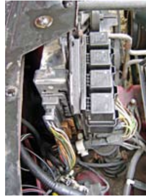
Early lamp modules can fail.
