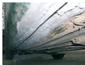
Sills should be solid rather than patched.
